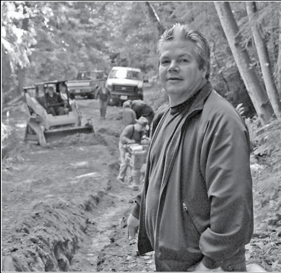
Yurok Public Utilities Manager and Yurok tribal member Rob Nulph oversees the installation of 5,000 feet of HDPE intake line on Ke'pel water system.
