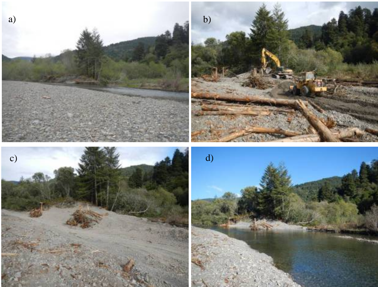
Figure 4. Photographs of ELJs 3-4 constructed during 2012 in Terwer Creek, Lower Klamath River (Site: TC ELJ3-4A; Photo dates: a) 4/24/12, b) 10/20/12, c) 10/21/12, d)10/25/12).
