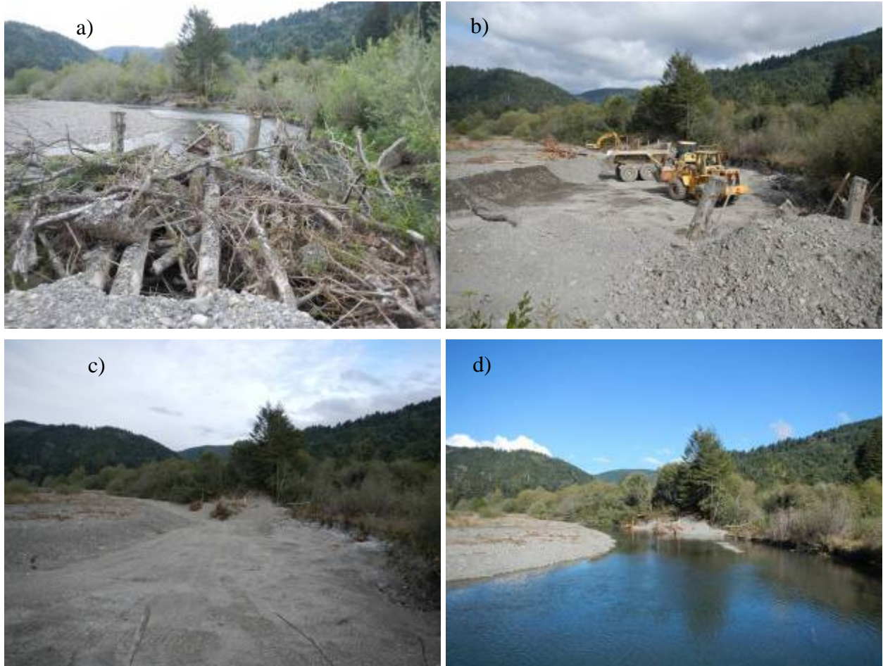
Figure 5. Photographs of ELJs 3-4 constructed during 2012 in Terwer Creek, Lower Klamath River (Site: TC ELJ3-4B; Photo dates: a) 4/24/12, b) 10/20/12, c) 10/21/12, d)10/25/12).
