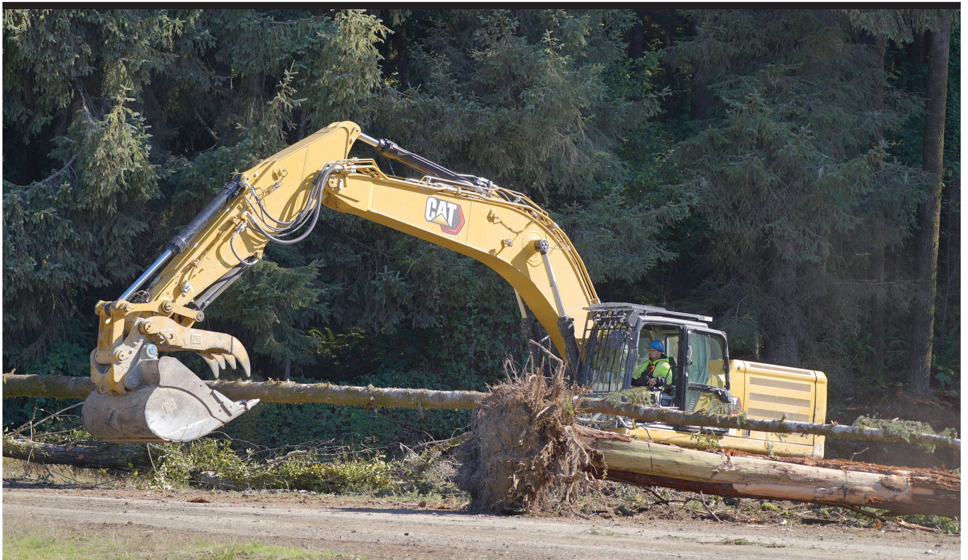
DANIEL MCQUILLEN , YUROK TRIBE CONSTRUCTION CORPORATION, PARTICIPATED IN THE PRAIRIE CREEK PROJECT.
