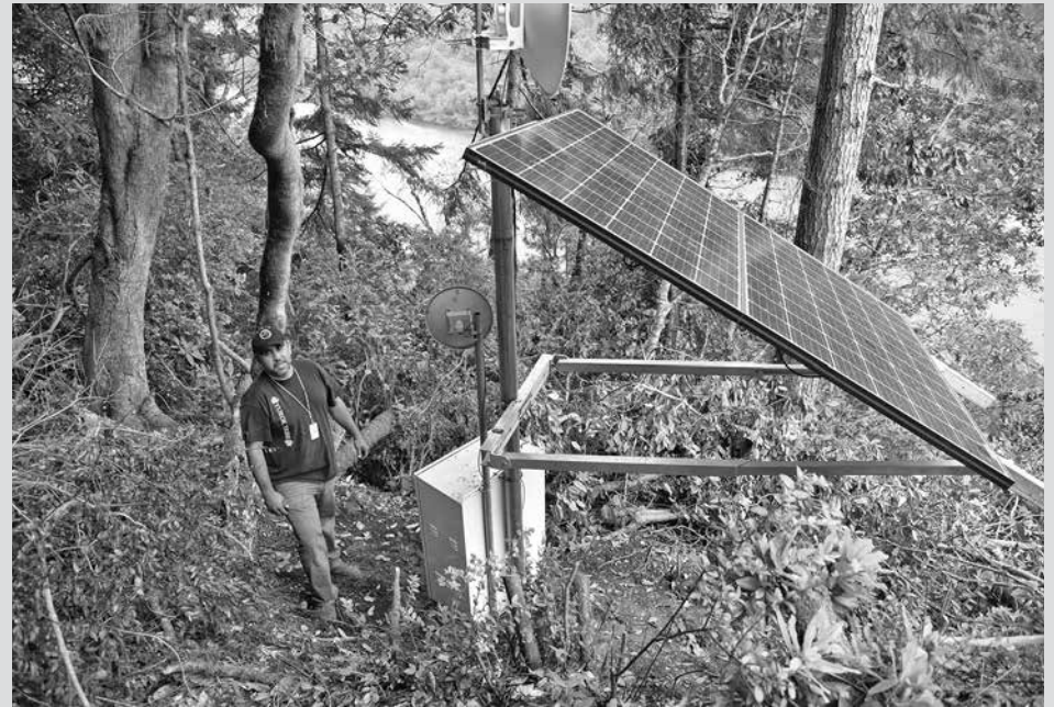
Broadband Technician Walter Hoffman, a Yurok Tribal member, stands next to the new relay site, which he helped install and sits on the south side of the Klamath River.
