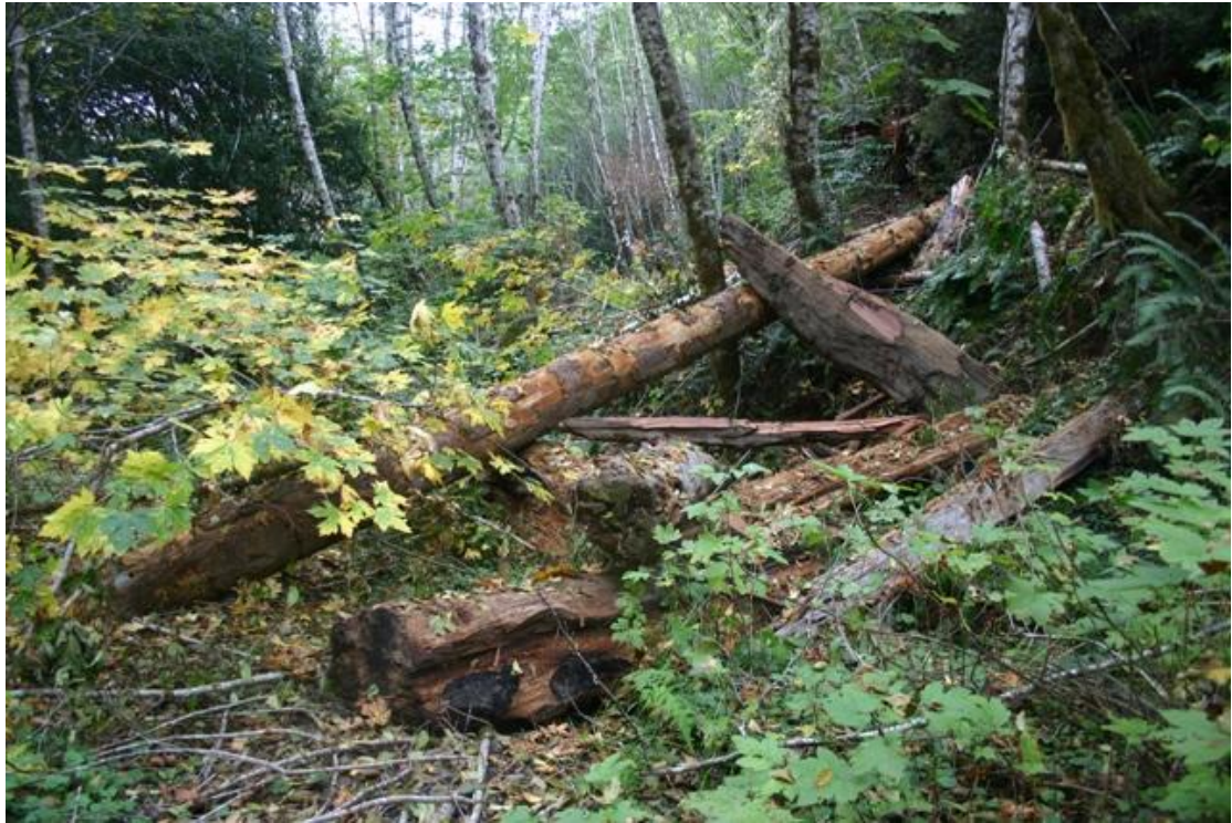
Figure 113. Lower end of LWD placement reach following installation of structure #20, Mainstem McGarvey Creek, Lower Klamath River, California, October 2008.
