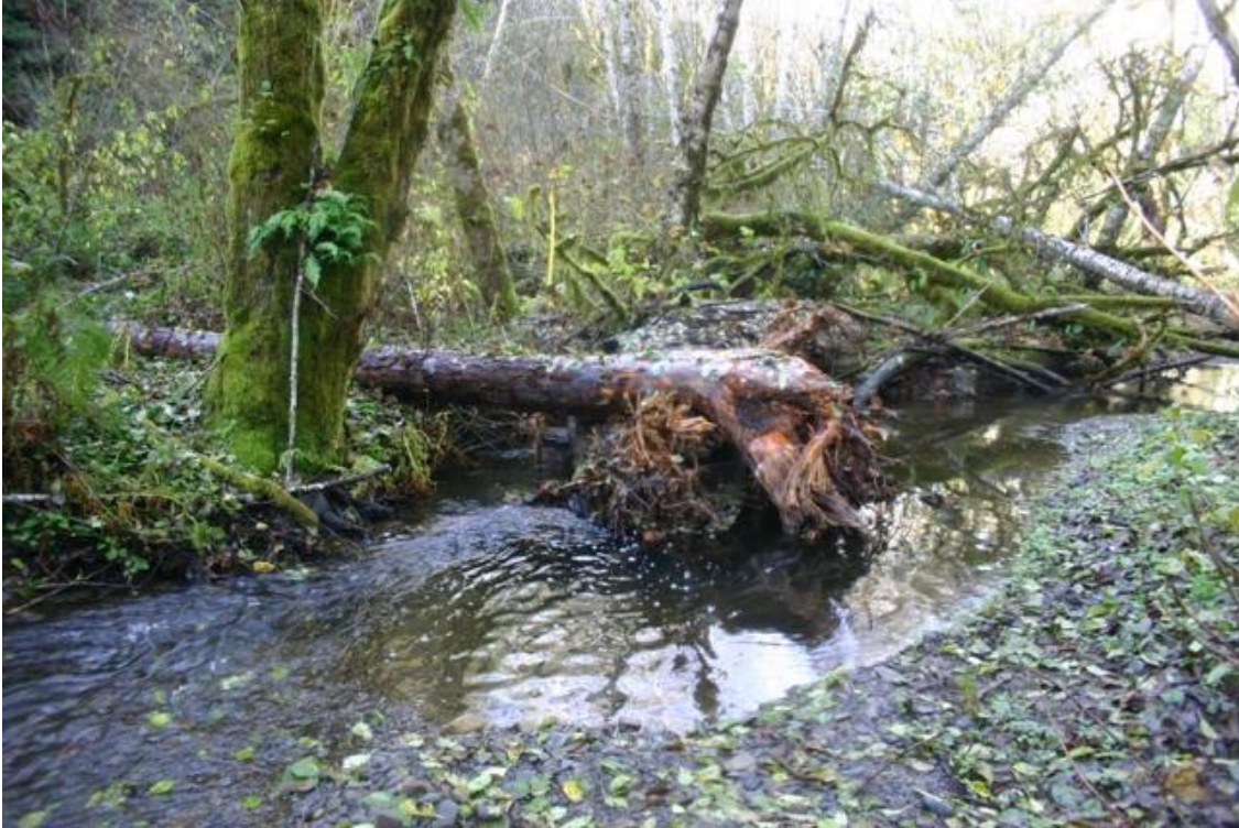
Figure 106. Scour pool habitat following installation of structure #19, Mainstem McGarvey Creek, Lower Klamath River, California, November 2008.
