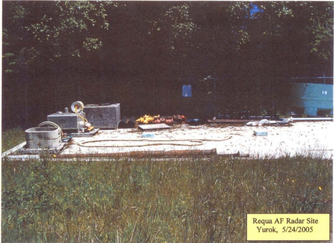
Standing at the entrance road at the west portion of the radar site and looking east towards the northern end of the removed Building 106 concrete pad and the radar site boundary fencing. The equipment on the concrete pad is temporarily stored equipment from National Parks Services and will be removed.
