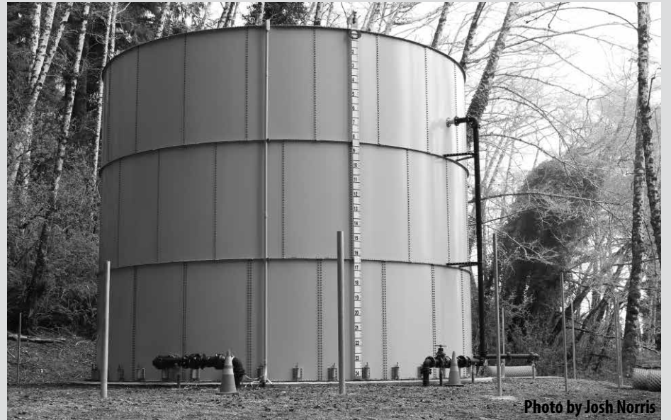
This tank has a 100,000 gallon carrying capacity and will provide dependable water security.
