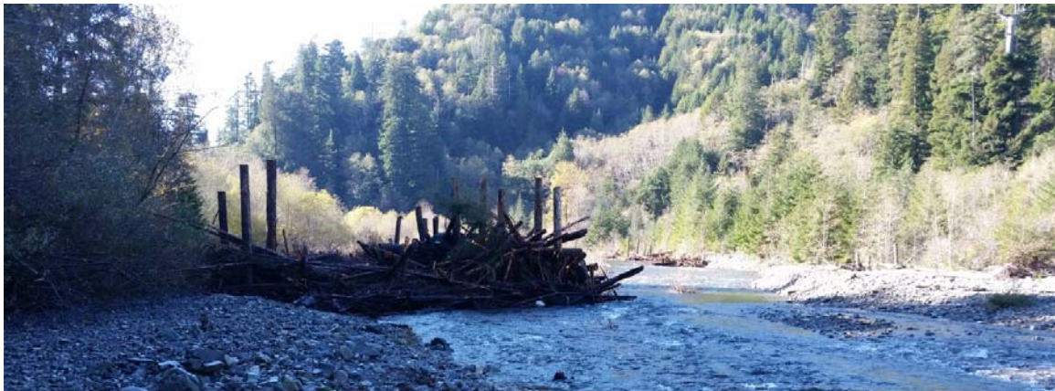
Figure 6. A bar apex jam in Terwer Creek prior to construction (Top – March 2016), during installation (Middle – October 2016), and post-construction (Bottom – December 2016).
