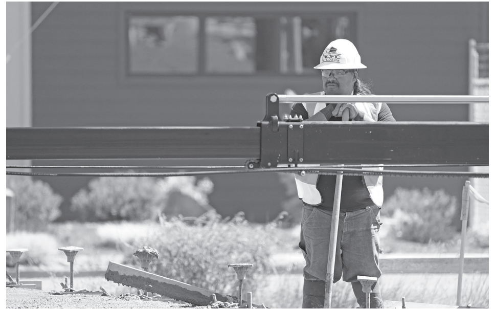
Yurok citizen John Donahue is a TERO placement working on the Emergency Operations Center project.
