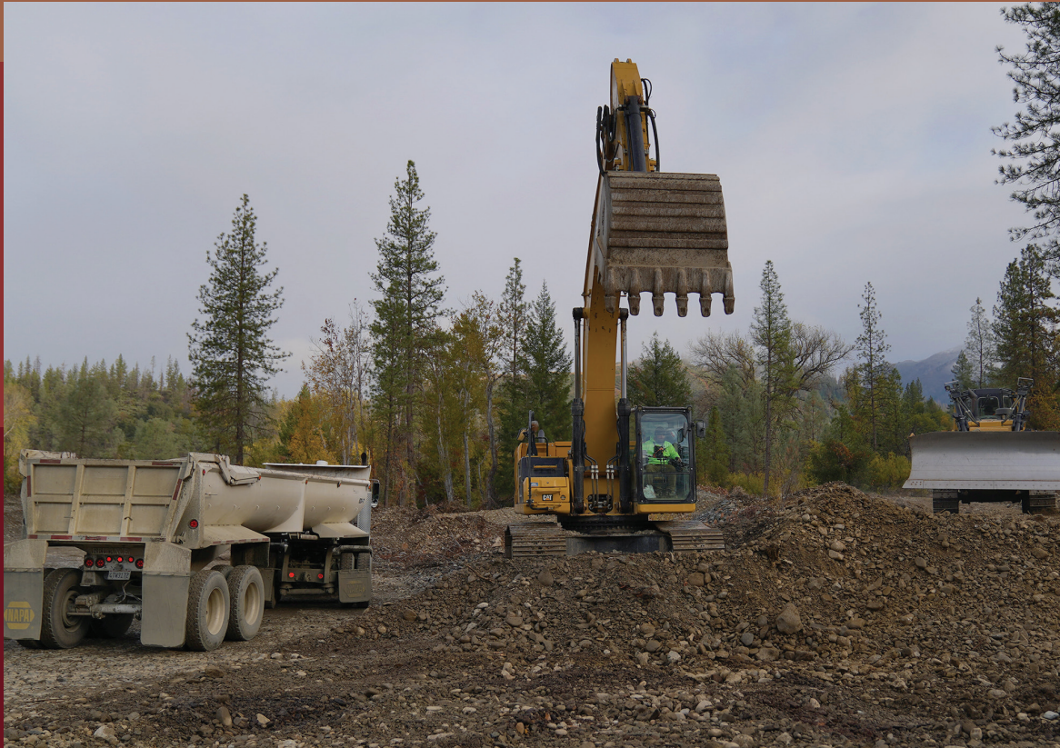
The Yurok Tribe Construction Corporation's remove historic gold-mining waste from the valley floor. The waste has impaired river function and harmed fish and wildlife for several decades.
