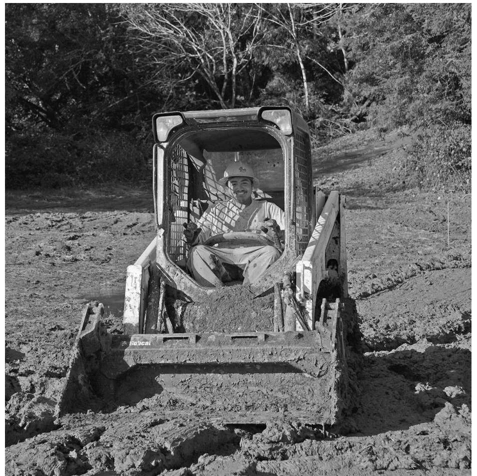
The Yurok Tribe Construction Corporation's Richard Bates works on the first pond.
