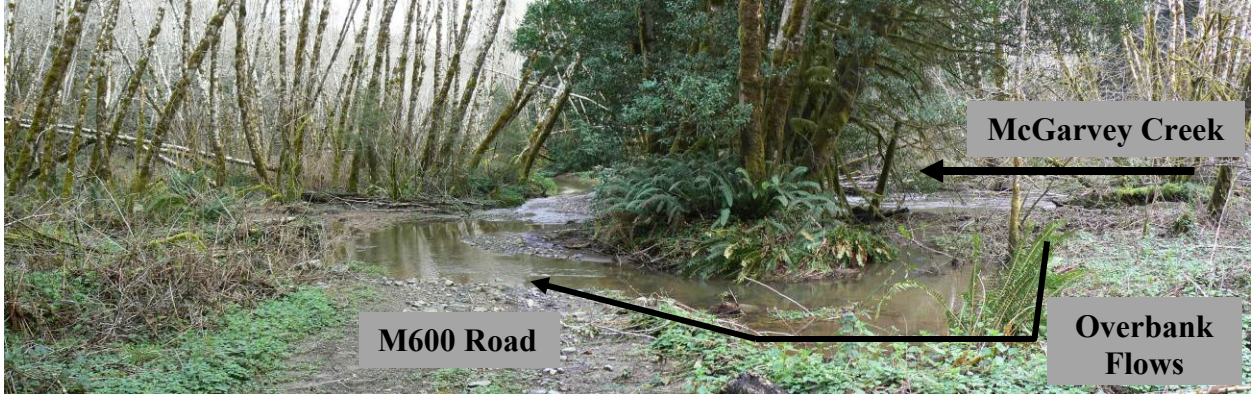
Figure 11. McGarvey Creek during an overbank flow event (note: flows onto M600 road 02/12/15).
