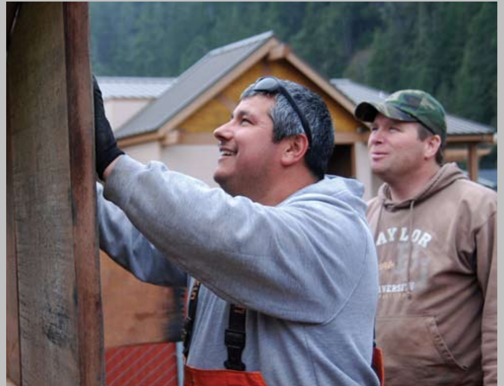
Tony Alameda puts up a redwood wall on a plank house at the Tribe's new Cultural Knowledge Park.
