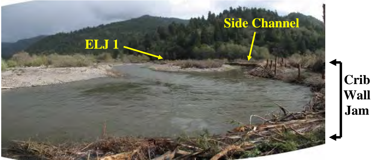
Figure 4. Looking upstream from Terwer Crib Wall Jam at Terwer ELJ1 and willow baffles protecting and creating complex slow velocity habitats for native salmonids (Winter 2010).
