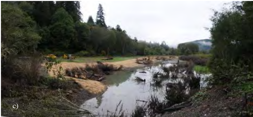
Figure 9. Photographs of Terwer Creek Pond B constructed during 2010 (Dates: a) 7/15/10, b) 7/28/10, and c) 10/31/10).
