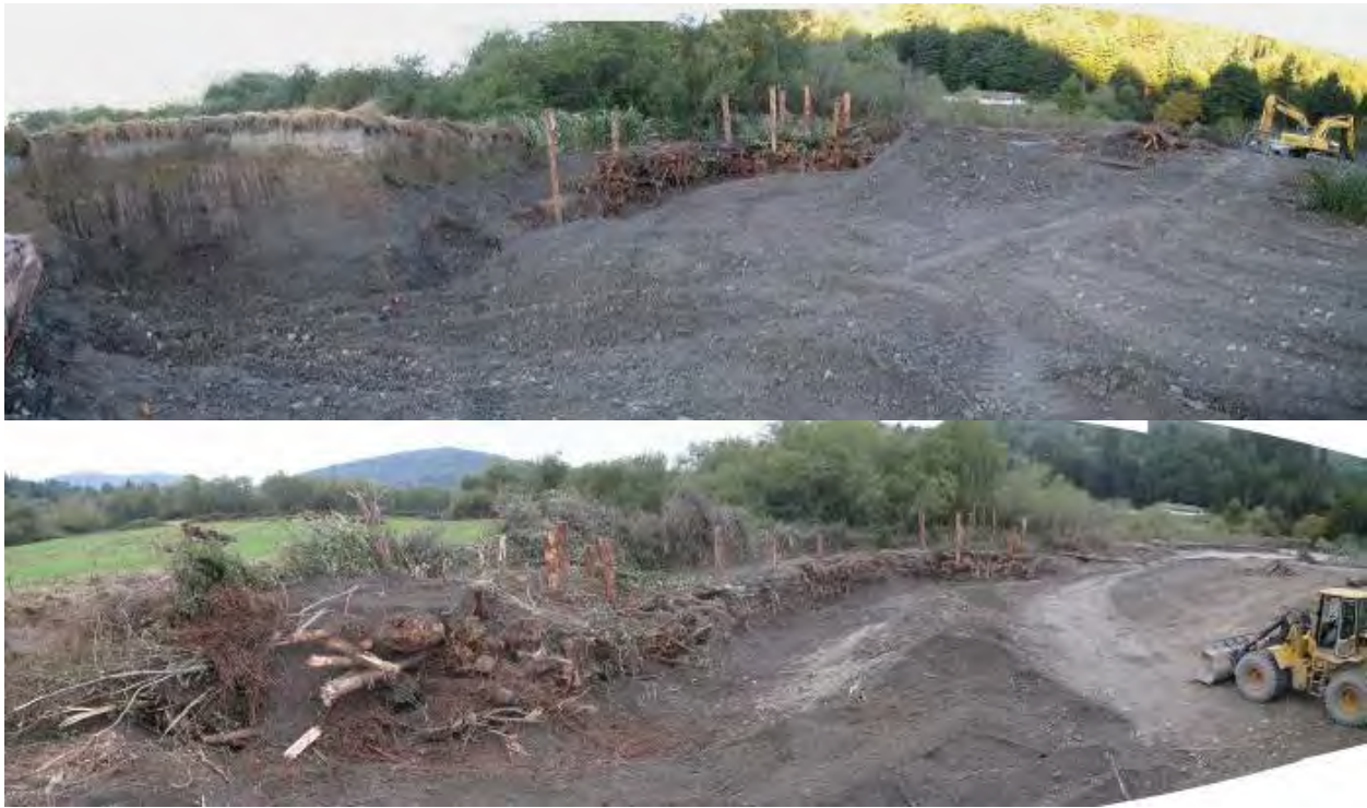
Figure 3. Looking downstream at an engineered log jam (Terwer Crib Wall Jam) in Terwer Creek during construction (Fall 2009).
