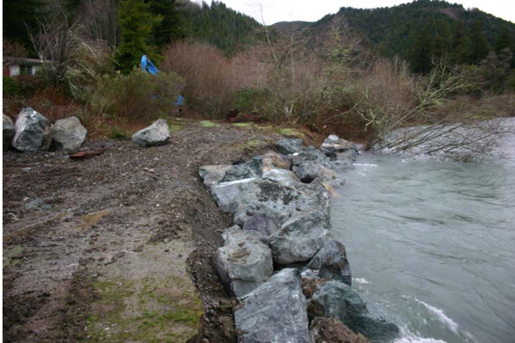
Figure 8. Upper half of project site during boulder placement, Lower Terwer Creek , Lower Klamath River, California, January 31, 2006.
