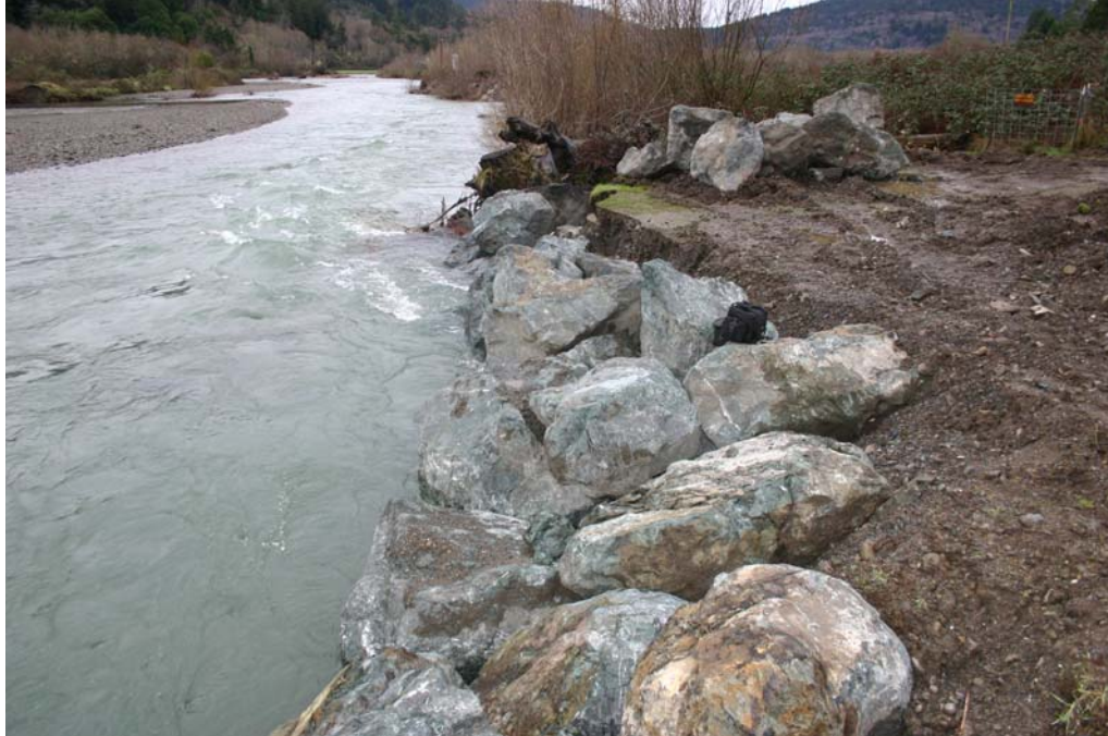
Figure 9. Lower half of project site during boulder placement, Lower Terwer Creek , Lower Klamath River, California, January 31, 2006.
