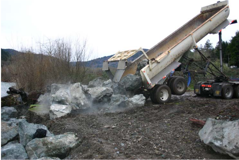
Figure 10. Boulders being delivered to project site, Lower Terwer Creek , Lower Klamath River, California, January 31, 2006.
