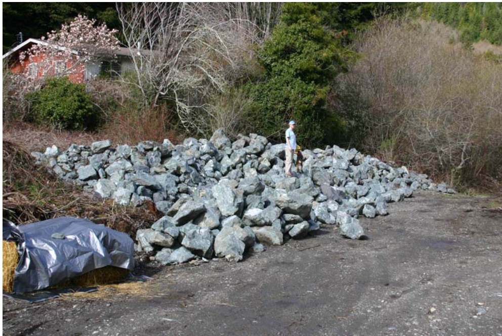
Figure 15. Stockpiled boulders at project site, Lower Terwer Creek, Lower Klamath River, California, February 28, 2006.
