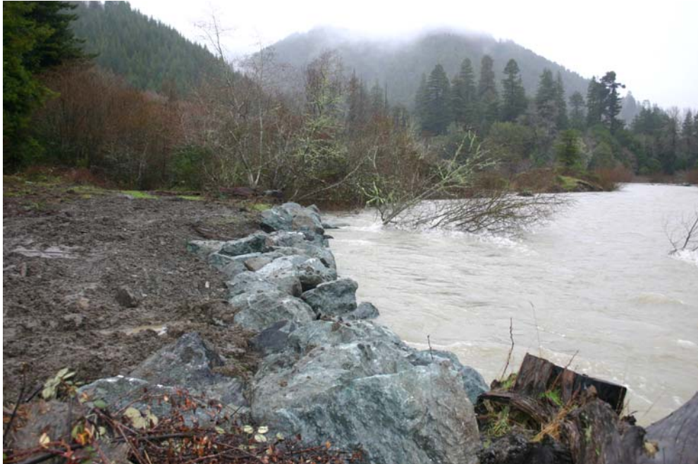
Figure 12. Stabilized streambank viewed from lower end of project site, Lower Terwer Creek ,Lower Klamath River, California, February 01, 2006.
