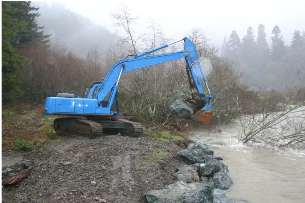
Figure 11. Excavator placing boulders at project site, Lower Terwer Creek , Lower Klamath River, California, February 01, 2006.
