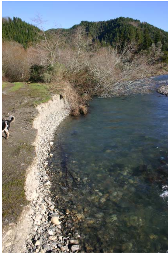
Figure 6. Streambank erosion at project site, Lower Terwer Creek , Lower Klamath River, California, January 24, 2006.
