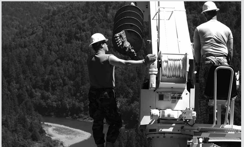
Military contractors construct one of the first sections of the power line.
