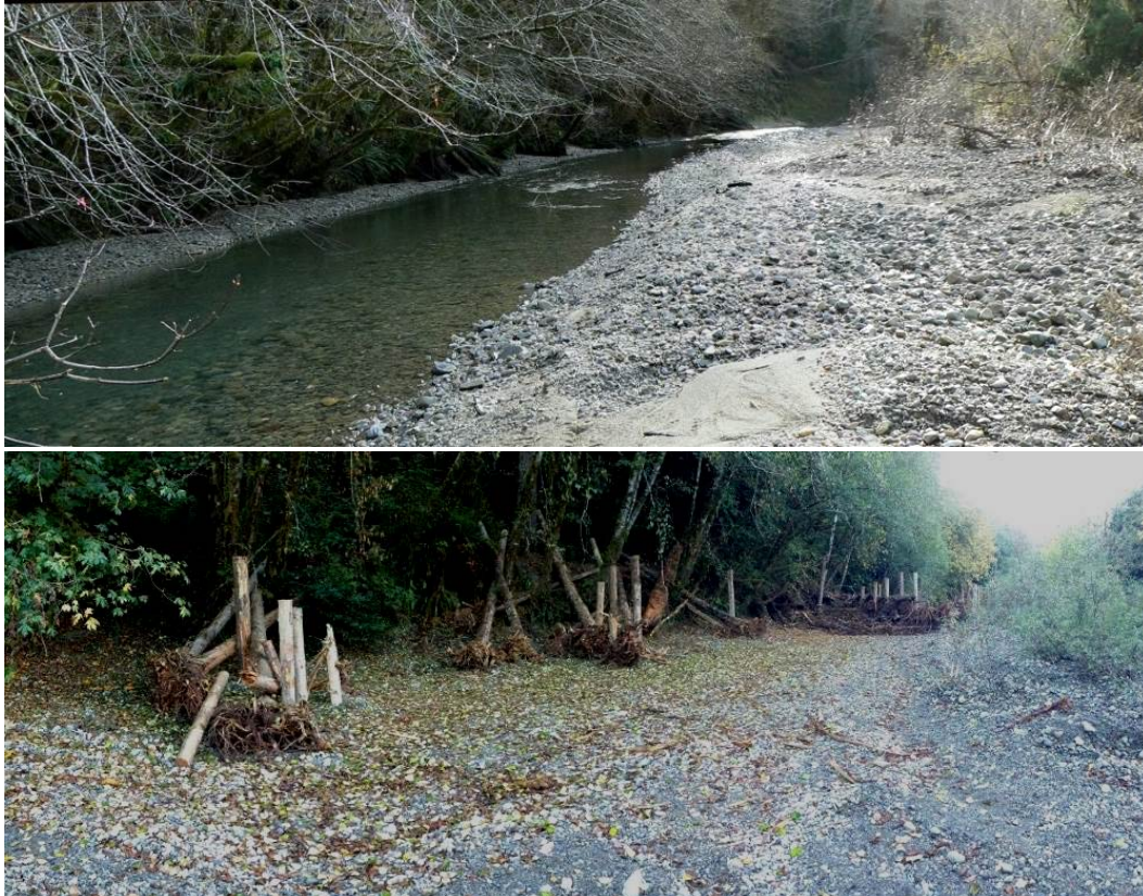
Figure 4. A constructed wood jam site in Hunter Creek prior to installation (Top – 01/18/15) and as-built (Bottom – 10/24/15).
