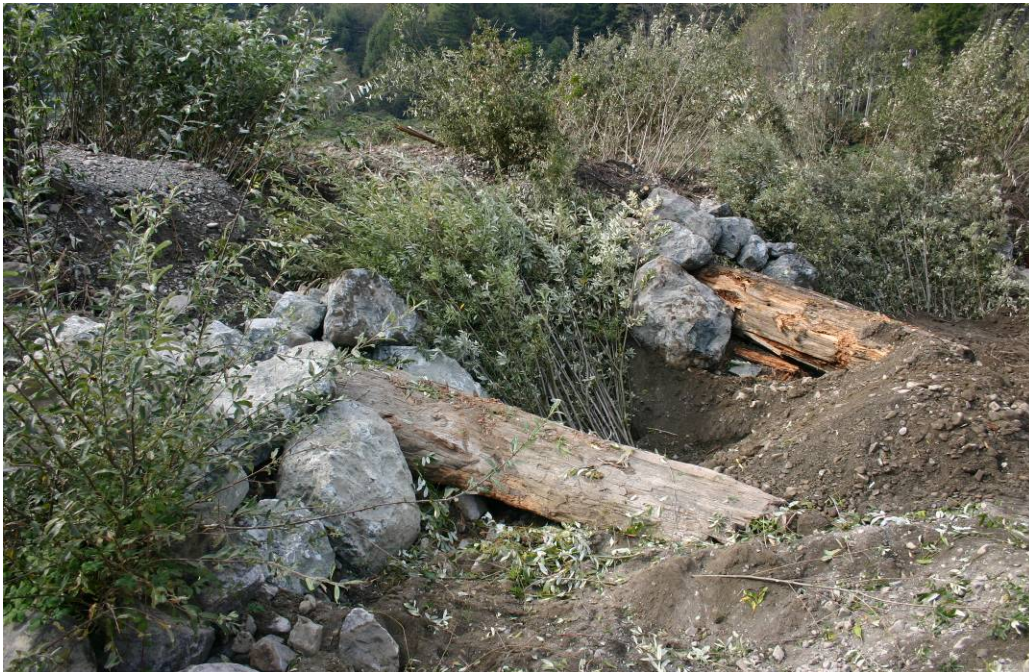
Figure 22. Installing willow mattresses between log-boulder structures, Lower Terwer Creek, Lower Klamath River California, 2005.
