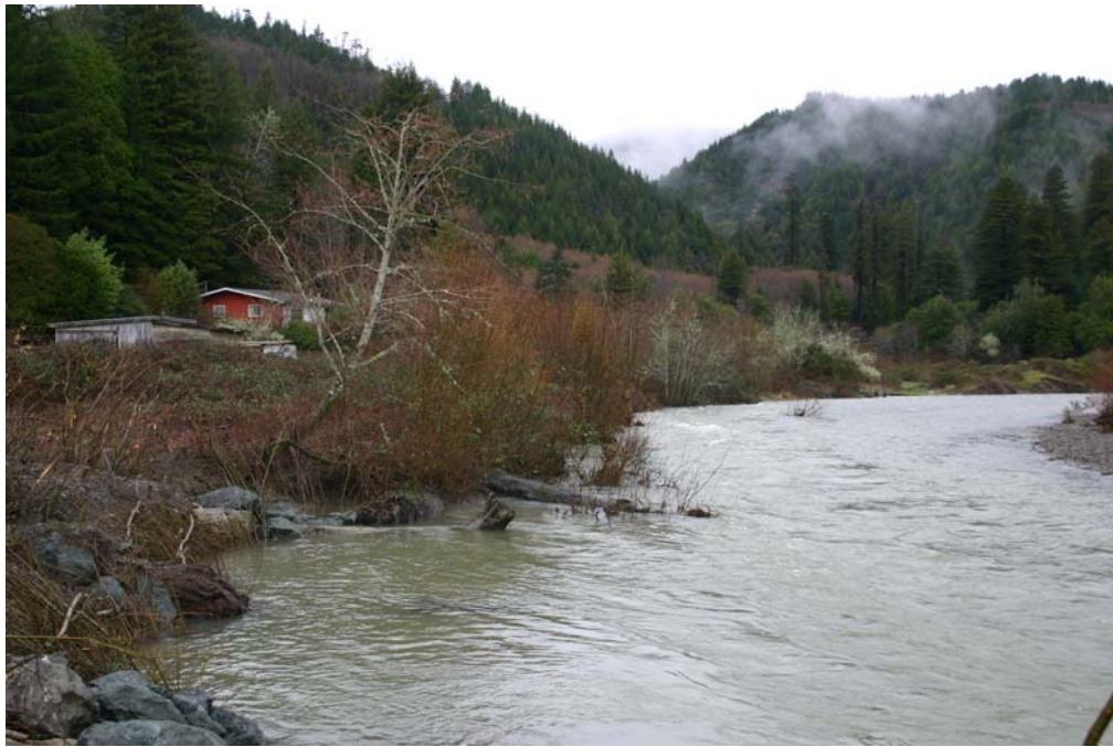
Figure 25. Boulder-log bank stabilization structures under increased streamflows, Lower Terwer Creek, Lower Klamath River, California, January 20, 2006.
