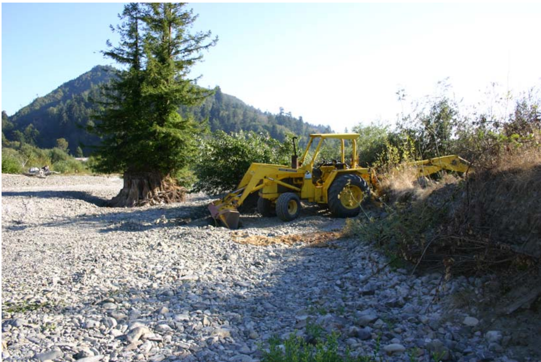
Figure 8. Excavating willow siltation baffle trench at lower end of baffle/mattress project site, Lower Terwer Creek, Lower Klamath River, California, 2005.
