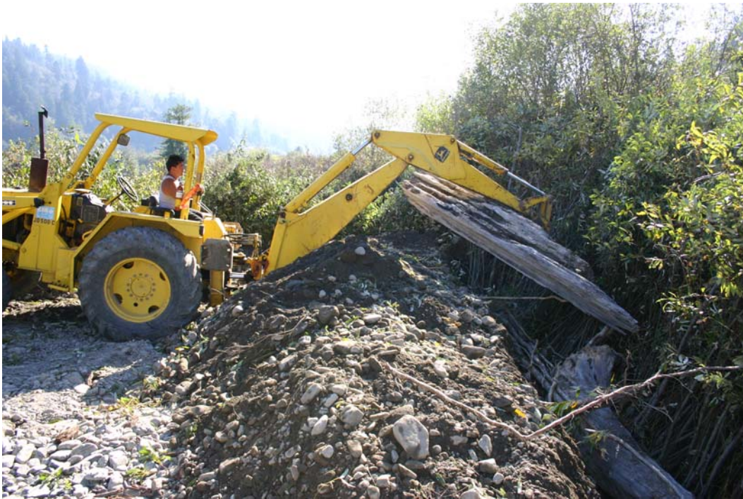
Figure 13. Placing LWD in willow mattress trench, Lower Terwer Creek, Lower Klamath River California, 2005.
