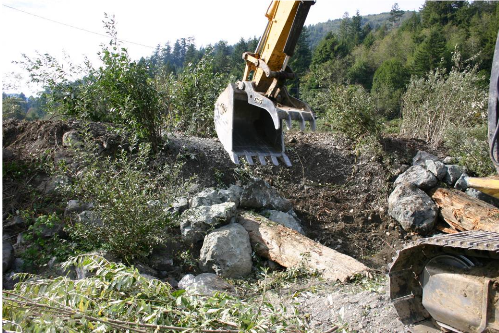
Figure 21. Installing boulders on log-boulder bank stabilization structures, Lower Terwer Creek, Lower Klamath River California, 2005.
