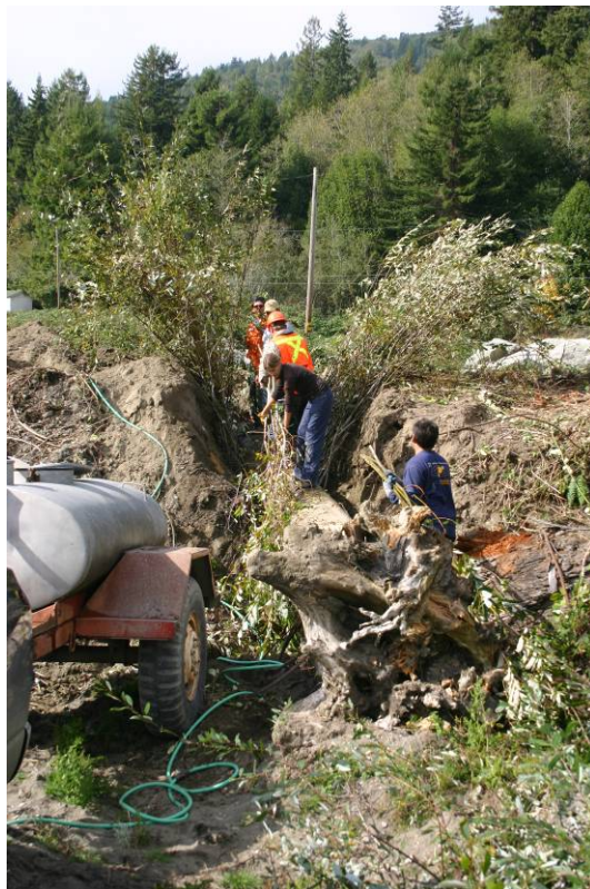
Figure 20. Planting willow cuttings in log-boulder bank stabilization structures, Lower Terwer Creek, Lower Klamath River California, 2005.
