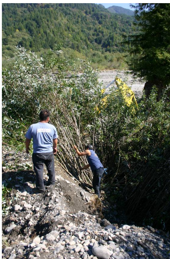
Figure 10. YTFP staff constructing willow siltation baffle, Lower Terwer Creek, Lower Klamath River California, 2005.
