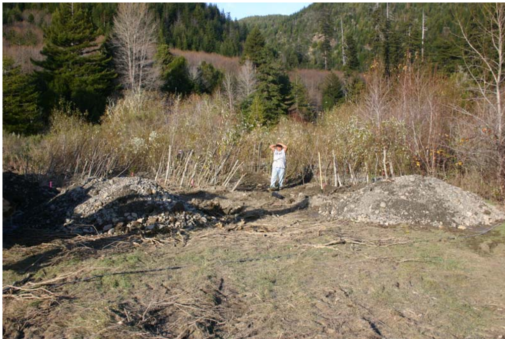
Figure 26. YTFP staff installing willow baffles on adjoining flood terrace, Lower Terwer Creek, Lower Klamath River, 2005.
