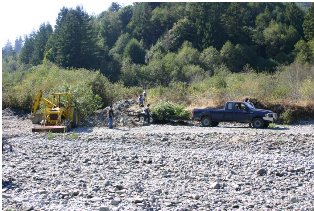
Figure 9. YTFP staff constructing willow siltation baffle, Lower Terwer Creek, Lower Klamath River California, 2005.
