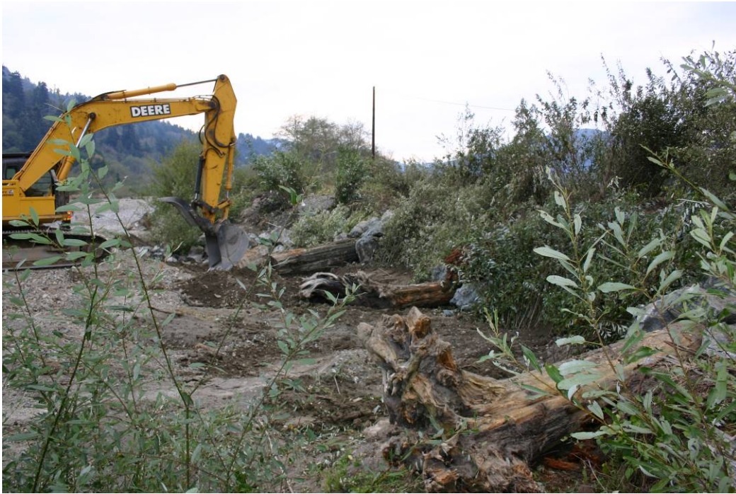
Figure 23. Completing finishing touches on bank stabilization site, Lower Terwer Creek, Lower Klamath River, California, 2005.
