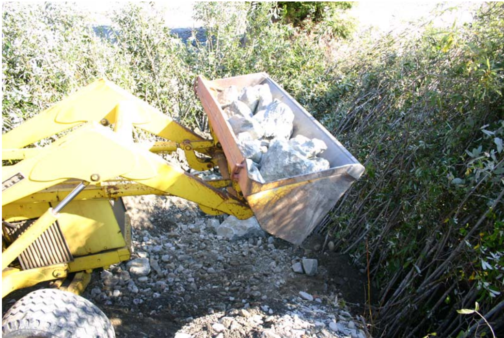
Figure 12. Placing quarter-ton quarry rock on willow siltation baffle, Lower Terwer Creek, Lower Klamath River, California, 2005.
