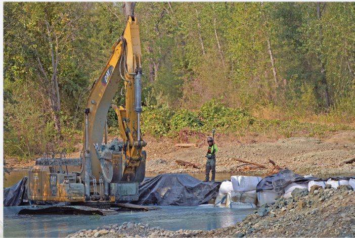
The Yurok Fisheries Department's Charlie Moon uses a digital device to guide the construction of new salmon habitat.
